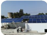
Solar Rooftop Plant
