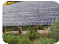
Ground-mounted Solar Power Plant
